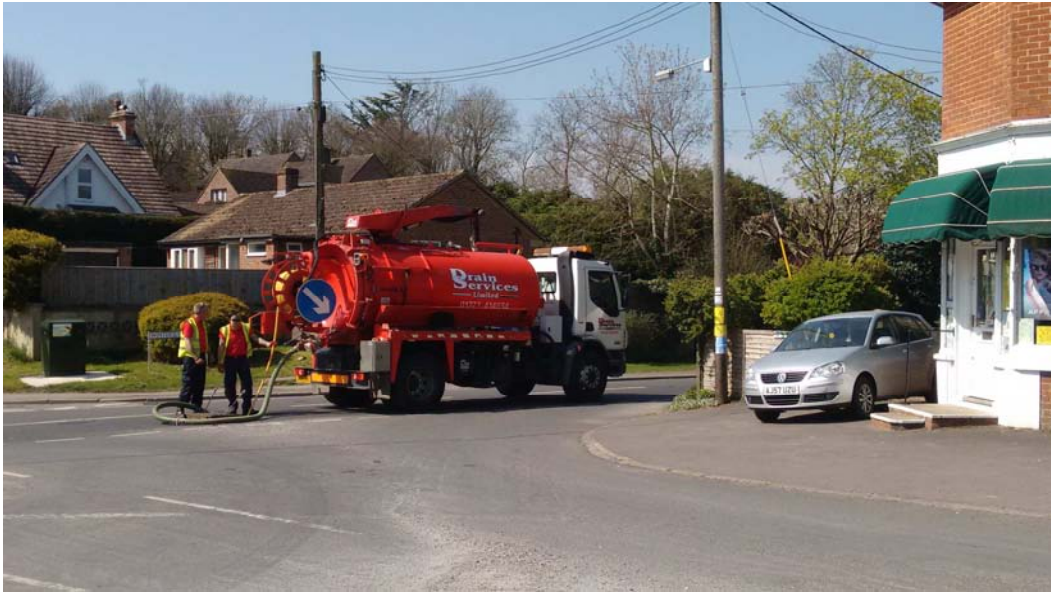
5— Frequent cleaning of drains and gullies may suggest siltation problems with drains in Porton High Street.
